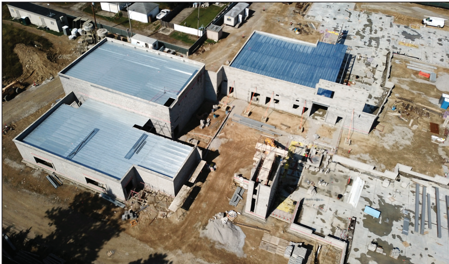
The new Hamilton Elementary School under construction on Middle Avenue and 13th Street.
