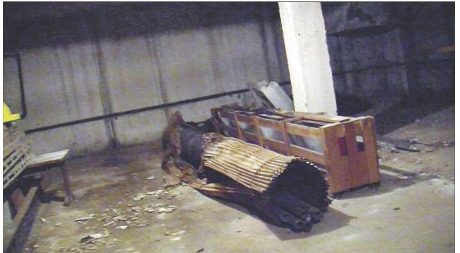
Parts of Ely Elementary's basement are unusable because of water damage.
